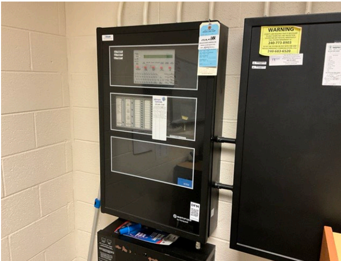
15 - FIRE ALARM PANEL
